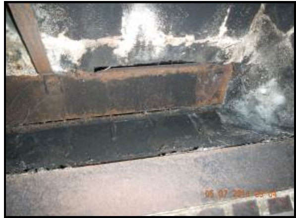
Efflorescence and damage
