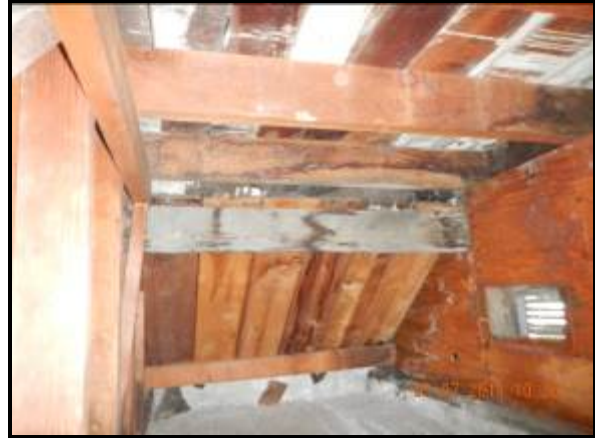
Stains on framing below porch
